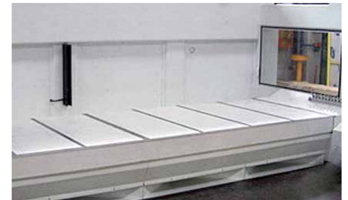
Dust extraction vents
